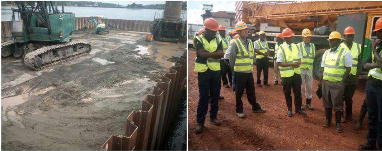
Figure 3.8: Left is the pile on the Kampala side which is about 85% complete and Right is the NPA staff and the project team
