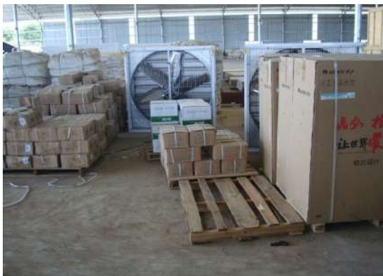
Figure 9: Goodwill Uganda Ceramic Ltd Equipment awaiting installation
