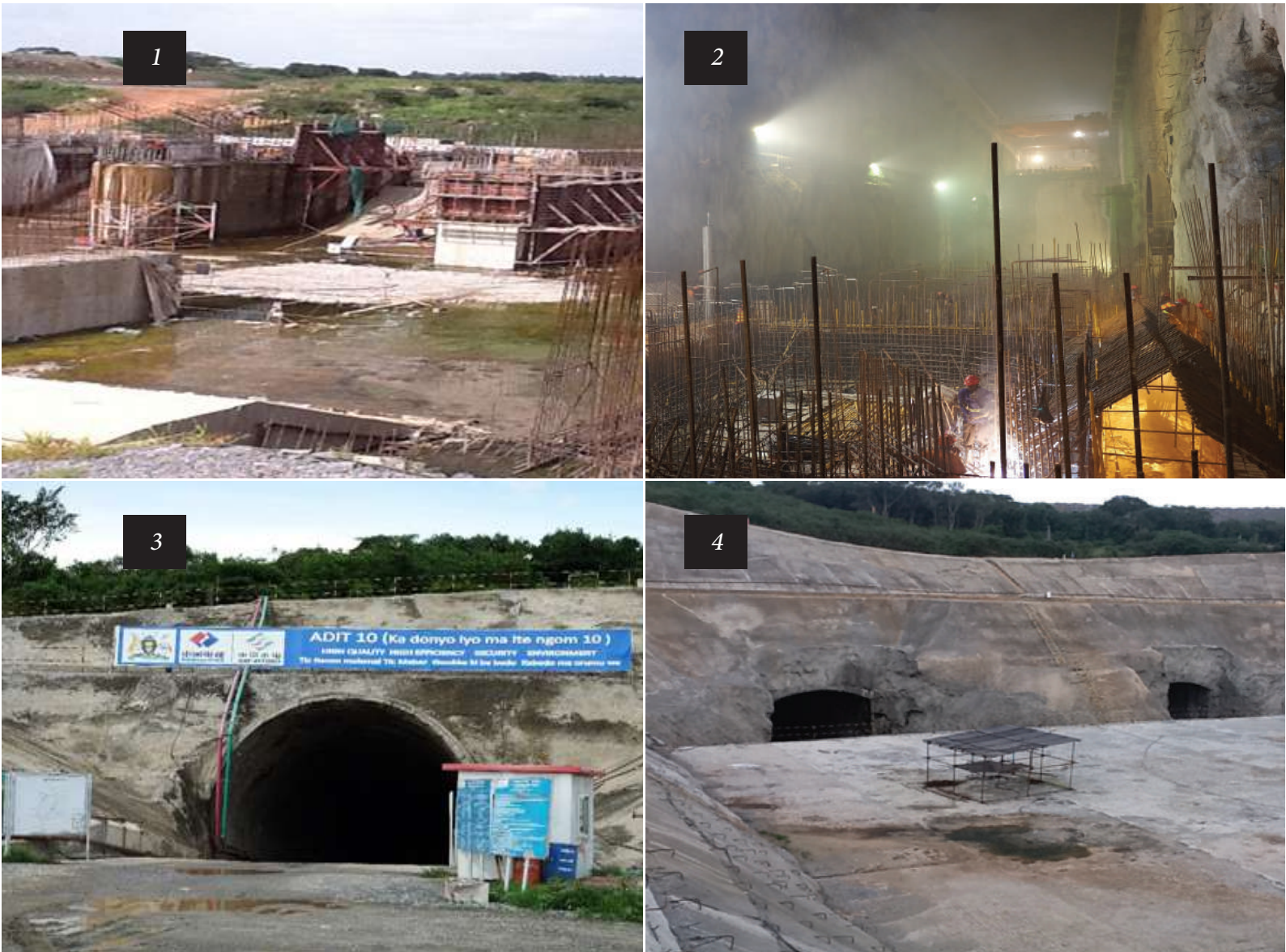
Figure 3.5: Pictures highlighting the progress of Karuma Dam construction (1) Construction of spillway (2) Construction of underground power House (2) Access for Tunnel construction (3)Tailrace Tunnel outlet
